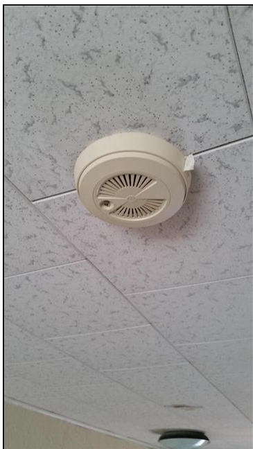
6.7 Item 1(Picture) Smoke detector in 2nd floor is an older model and should be replaced.
