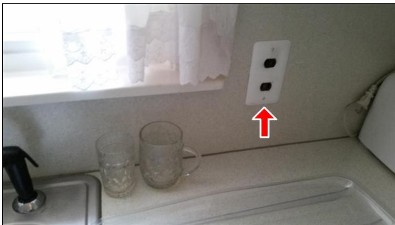
6.4 Item 2(Picture) Standard receptacle (not GFCI) too close to water source.
