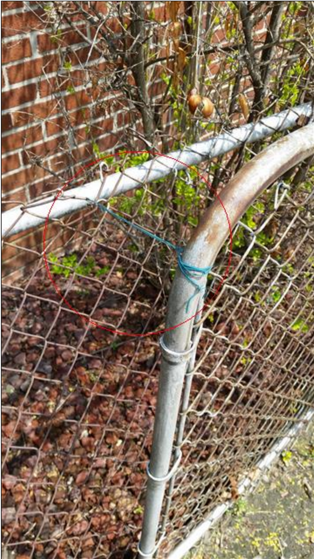
2.5 Item 1(Picture) North portion of driveway gate is fastened to the fence.
