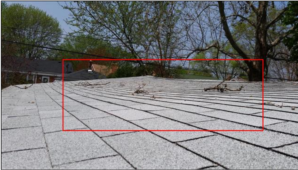
10.0 Item 1(Picture) Area of garage roof is slightly concave.
