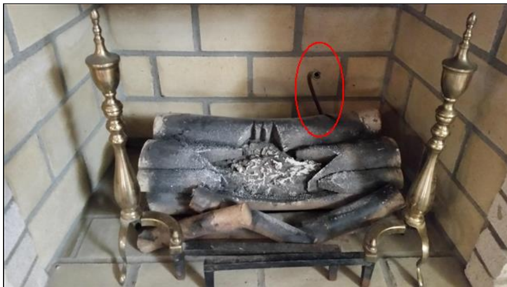
7.0 Item 1(Picture) Natural gas line is not correctly hooked up or positioned for fireplace use.
