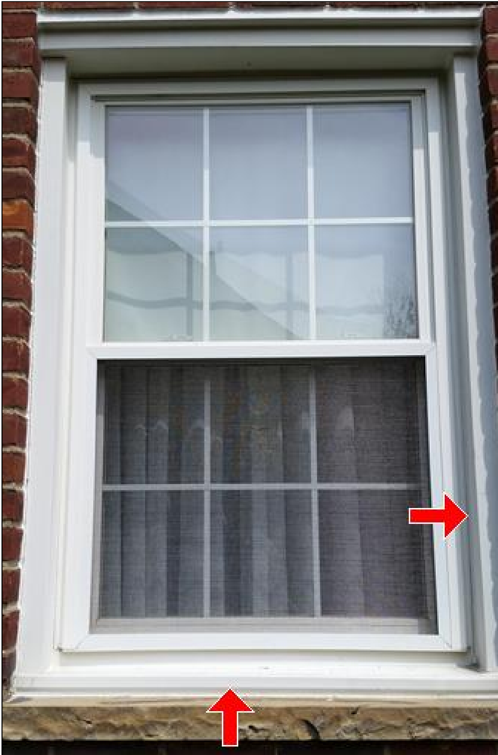
2.7 Item 3(Picture) Window seals are somewhat deteriorated.
