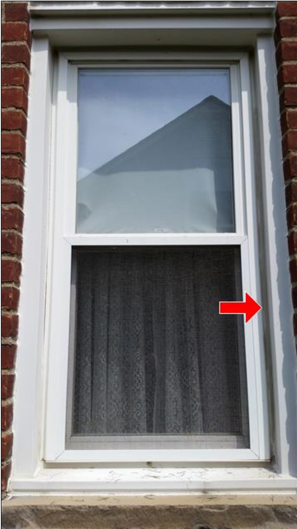
2.7 Item 4(Picture) Window seals are somewhat deteriorated.
