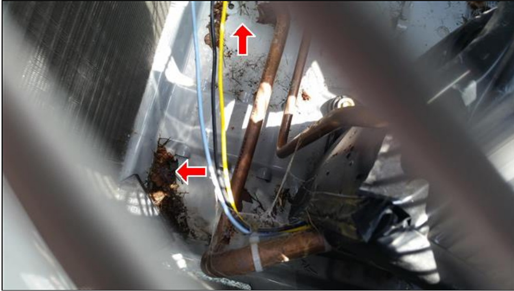
4.6 Item 2(Picture) awn debris noted in A/C unit.
