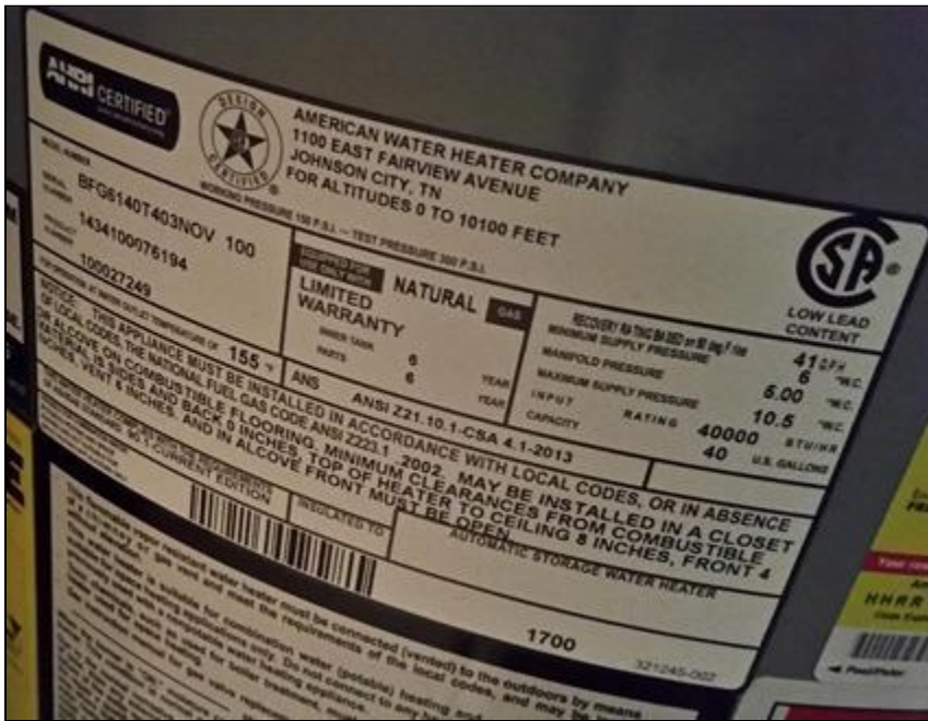
5.2 Item 1(Picture) Water heater info label.
