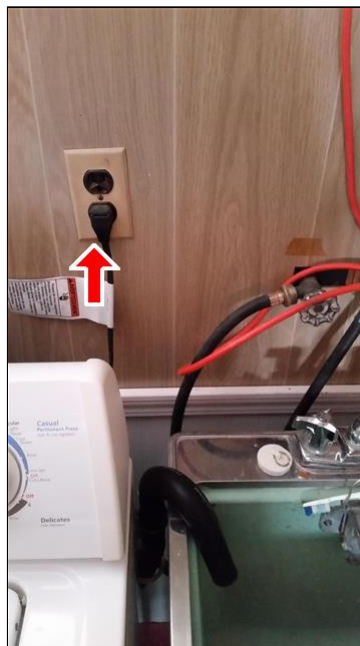
6.4 Item 3(Picture) Standard receptacle (not GFCI) too close to water source.
