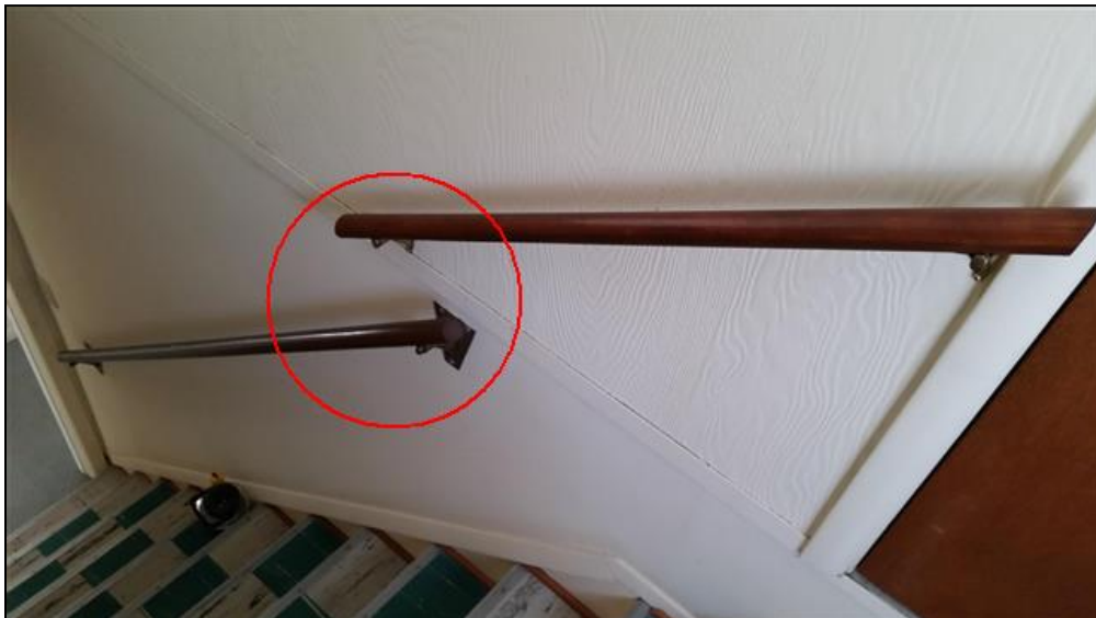
9.3 Item 1(Picture) Non-continuous railing to 2nd floor.
