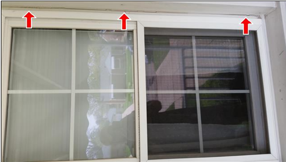
2.7 Item 5(Picture) Window seals are somewhat deteriorated.
