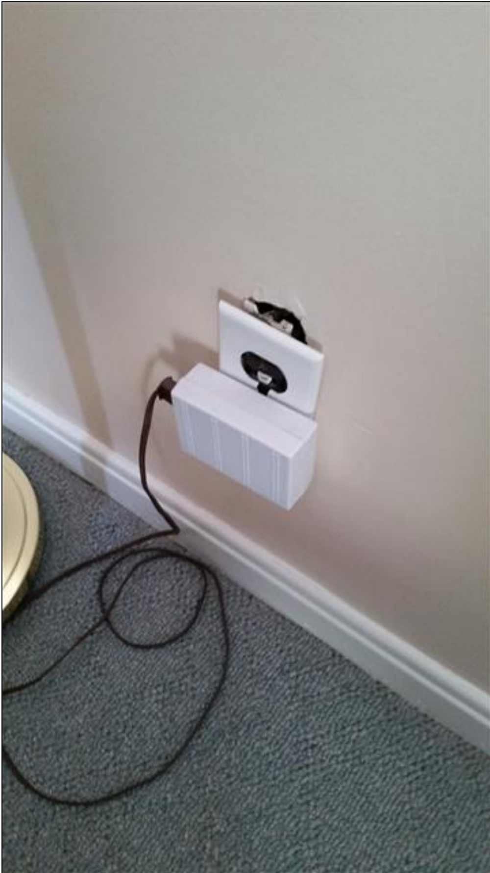
6.3 Item 1(Picture) Receptacle cover is broken.
