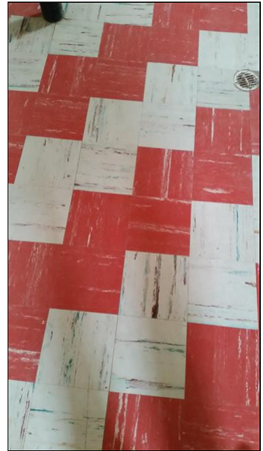
9.2 Item 2(Picture) Floor tile in basement may be of the asbestos type.
