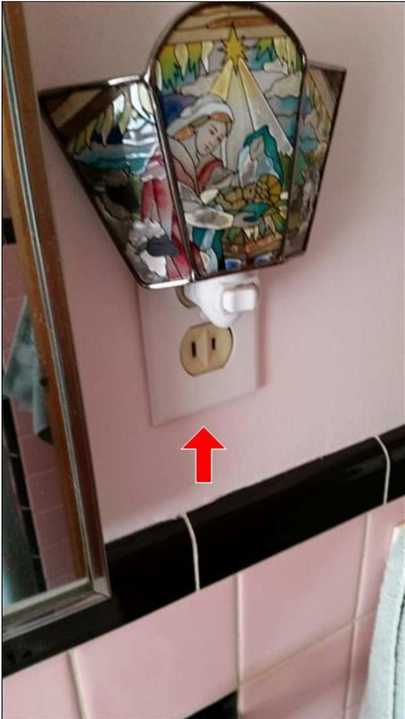
6.4 Item 1(Picture) Standard receptacle (not GFCI) too close to water source.
