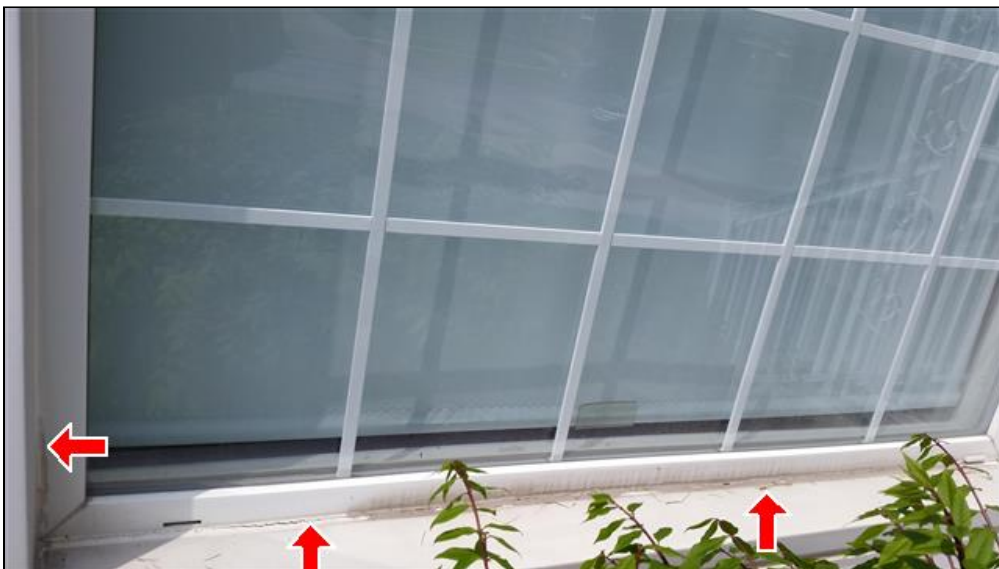
2.7 Item 2(Picture) Window seals are somewhat deteriorated.
