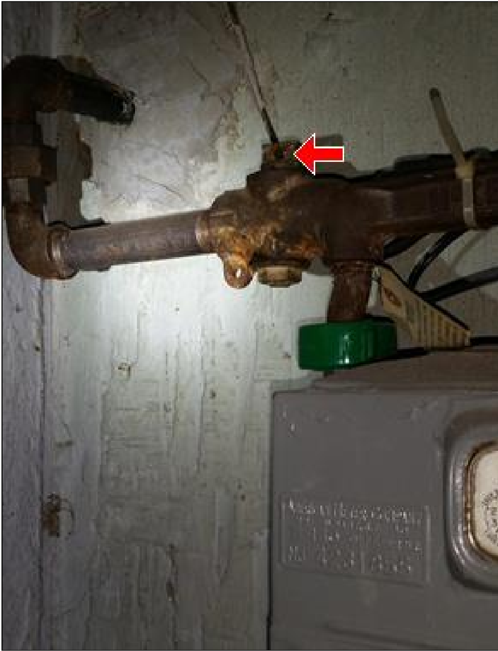
5.1 Item 2(Picture) Natural gas shut-off.
