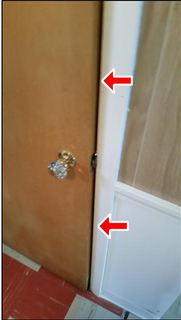
9.5 Item 1(Picture) Basement bathroom door does not close completely with pressure.
