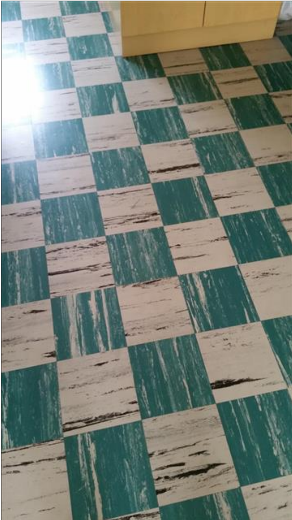
9.2 Item 1(Picture) Floor tile in 2nd floor may be of the asbestos type.
