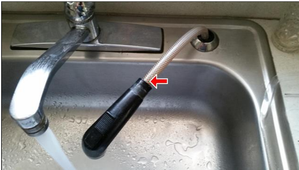
5.3 Item 1(Picture) Slight leak from kitchen sink spray attachment.
