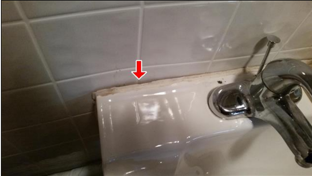
5.3 Item 2(Picture) Caulk bead behind basement bathroom sink is deteriorated.
