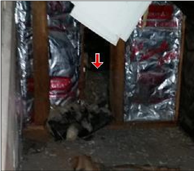
8.3 Item 1(Picture) Birds nest debris in the attic.
